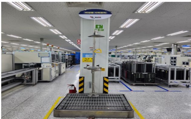
Emergency decontamination facility for hazardous chemicals
