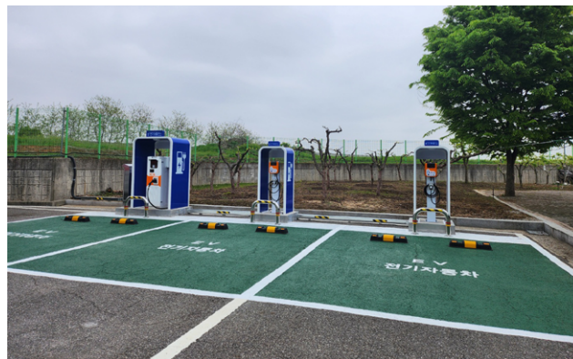
Electric vehicle charging facility
