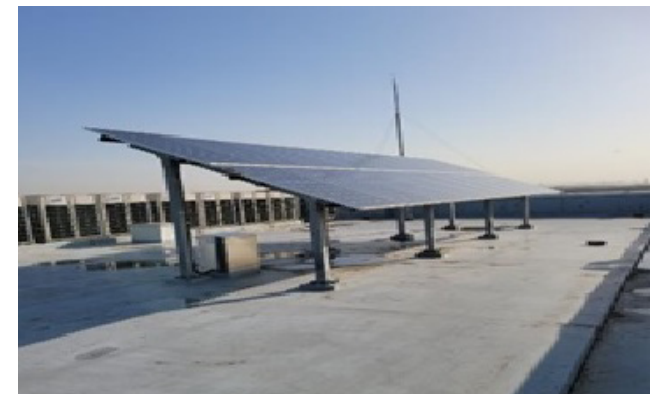
Solar power generation facility
