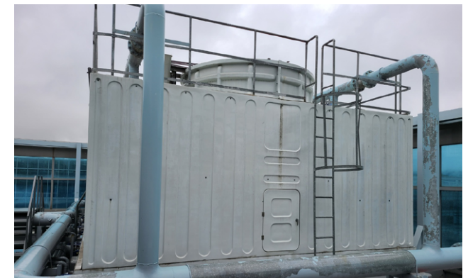
Cooling tower for water reuse
